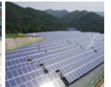
Solar Panel & Inverter
