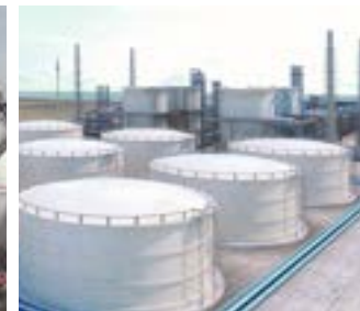
Atmospheric Storage Tank
