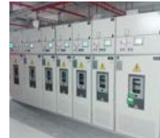
High Voltage Switch Gear
